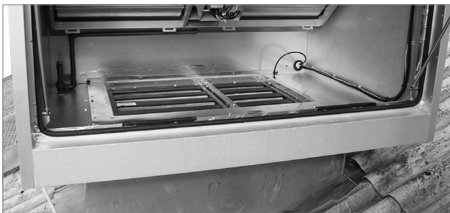
Fig. 28: Extract air filter installed in the unit
